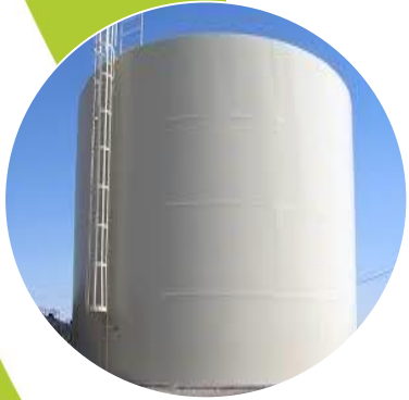
BioDiesel Storage Tank
